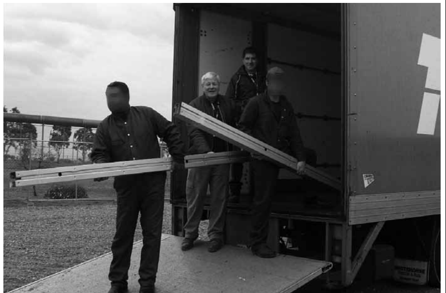
Noel Taylor and Owen Bayliss (second and third from the left) help inmates unload steel frames for the Habitat for Humanity project. The inmates' faces have been pixillated
